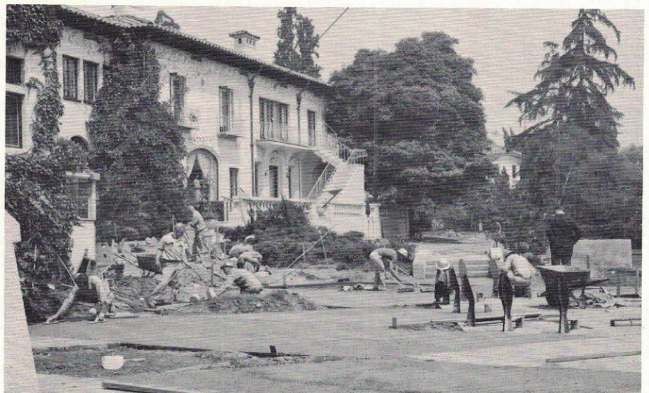
Here you see the beginning of a full day's work at pouring concrete. Students now can make full use of some very lovely facilities.
